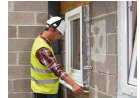
3. Position and secure the window unit and seal the external window/wall junction using Tyvek® Window Tape
