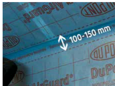
7. Apply AVCL, ensuring successive runs are adequately lapped to each other and onto adjacent wall surfaces
