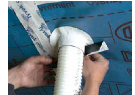
6. Apply a 2nd length of Tyvek® FlexWrap EZ onto the pipe on the opposite side. Try to keep the folded tape flat by 'pinching' together
