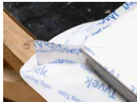
7. Form a loop on the corners: at least 1.5 x joint width - Repeat on all sides
