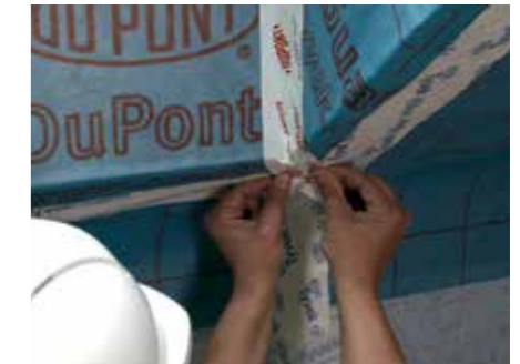
18. . . . a flexible tape that can be used to seal corners and any awkward details
