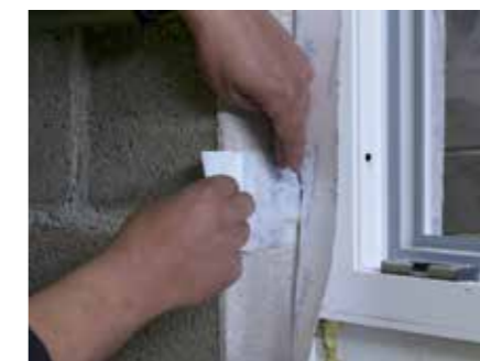
12. Apply Tyvek® Window tape to the window head and reveals taking care to seal and brackets.
