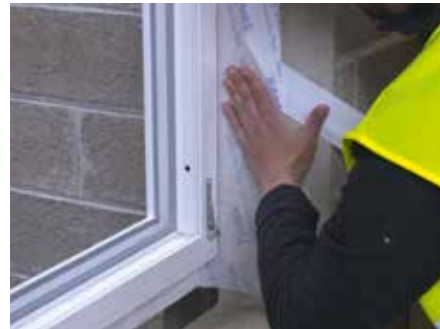
1. The internal window to wall junction can be sealed following the same method described on page 35
