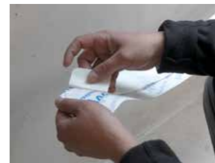
10. Peel away a short length of liner and apply the exposed tape onto the AVCL
