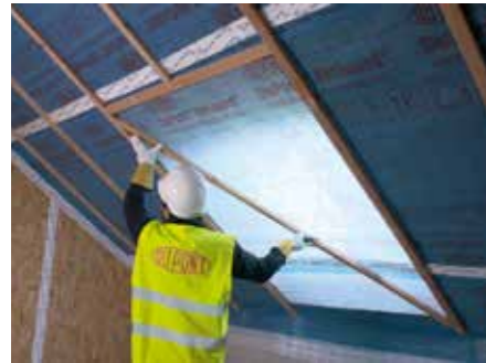
1. Cut a 'Y' into AVCL, using batten as a guide if preferred
