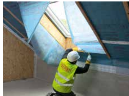
4. Cut AVCL horizontally across foot of window, in line with the reveal edge
