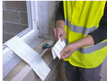
2. Internal corners can be sealed with a separate piece of Tyvek® Plastering Tape. Firstly, cut out a square of tape and fold in half
