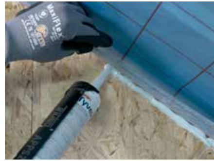
1. Whilst holding the DuPont™ AirGuard® AVCL back, apply a 4-8mm bead of DuPont™ AirGuard® Sealant to the surface
