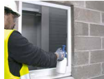
1. Spray water onto external surfaces to effect bond with DuPont™ Insta Stik™
