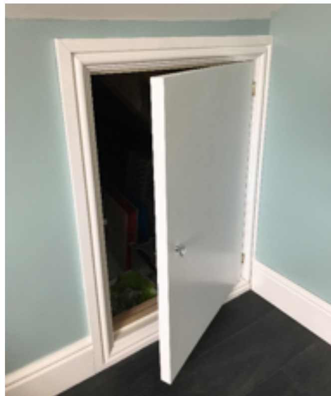
This eaves access door should have insulation and draught seals fitted
