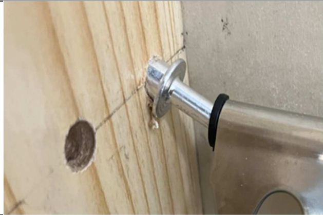
Exhibit #7. Damage detected
