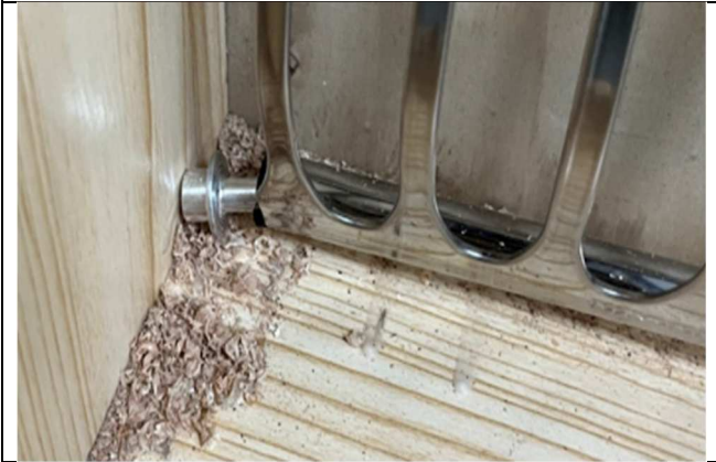
Exhibit #8. Damage detected
