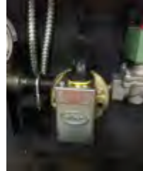
Low gas pressure switch failure
