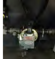
High gas pressure switch failure
