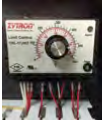
High temperature switch failure
