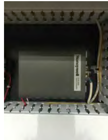
Ignition transformer: Check wire fitting connection
