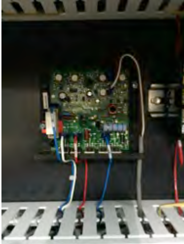
DC drive board connections
