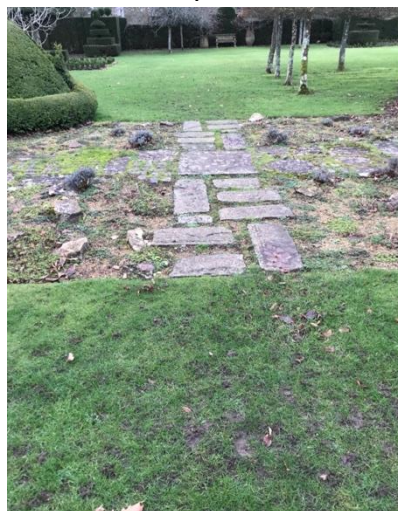
Uneven paving across Thyme Walk
