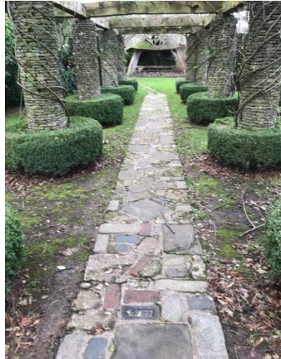
Uneven paving in the Pergola
