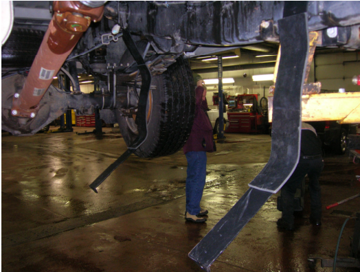
(Fig. 7) Carefully bend straps down out of the way in preparation for lifting tank into place.
