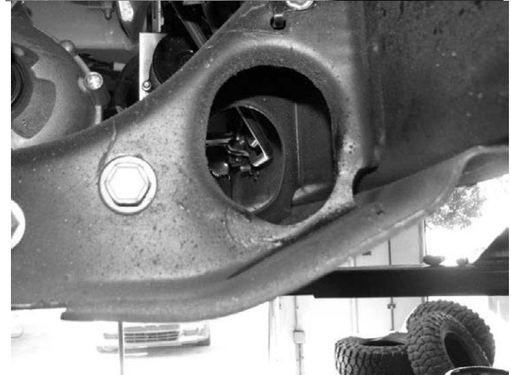
41. Locate and install the factory torsion bar through the hex in the torsion bar mount. Thread the torsion bar all the way back in the
