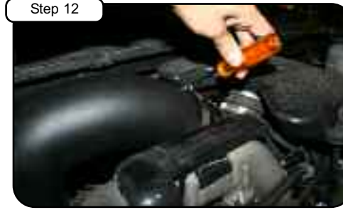
Step 12 Install 05-01072 tube to turbo side with 05-00632 reducer coupling and clamps provided and position to tube on housing. Do not tighten clamps.
