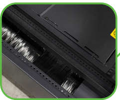
Brush cable managers in floor of cabinet
