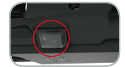
Main power switch
