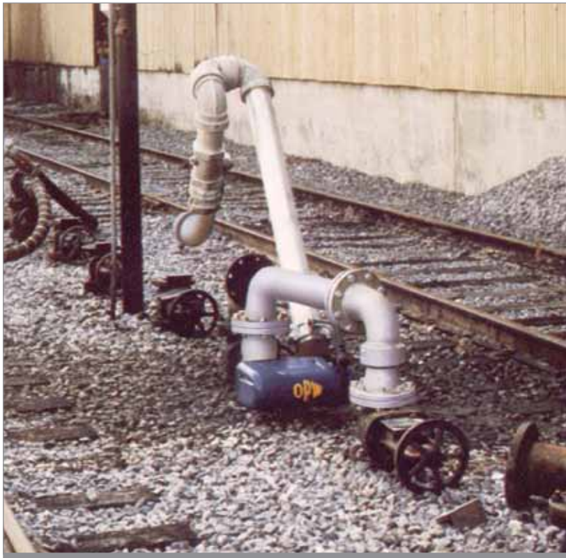
Swivel joints are an integral part of OPW's complete line of loading arm assemblies. This arm replaced hose in a railcar unloading operation.
