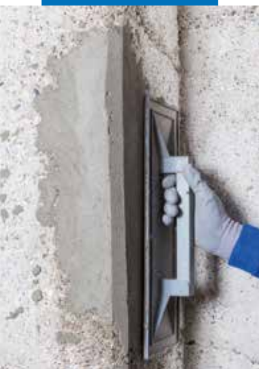
Floating the surface of Planitop Smooth & Repair R4 to create a smooth finish
