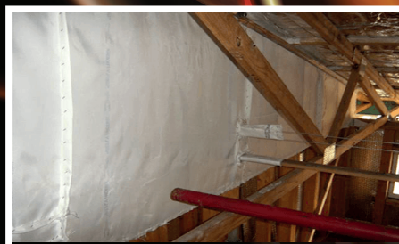
Age Care Centre Vertical Smoke/Flame Barrier
