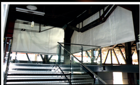
Smoke Reservoir at Finger Wharf, Walsh Bay, Sydney Harbour
