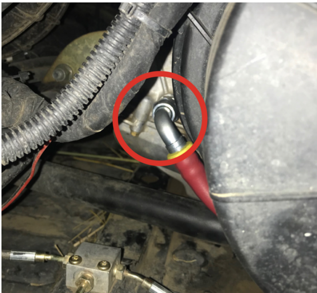
9. Install oil drain fitting into case and install new oil drain line
