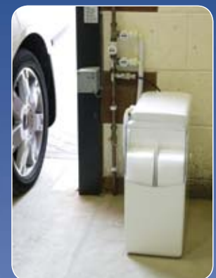
The TwinTec installed in the garage.
