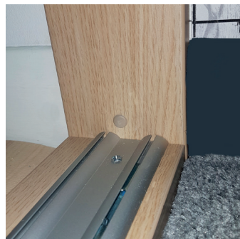
Skirting board cut out for strike plate
