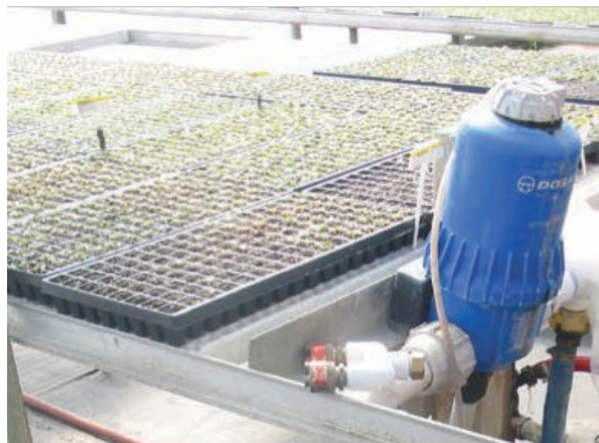
Dosatron injecting treatment solution into an irrigation boom.
