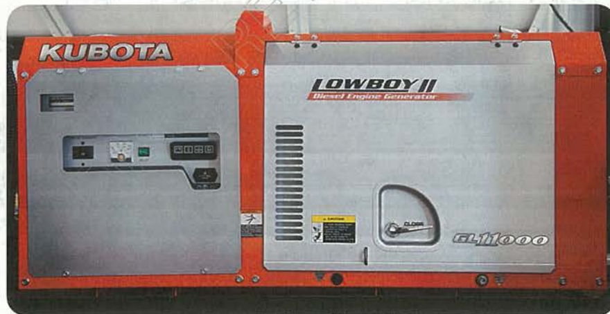
Figure 23 Kubota Diesel Generator
