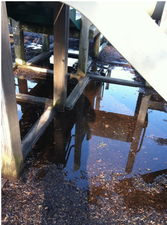
Bad drainage in Engineered Wood Fiber Install
