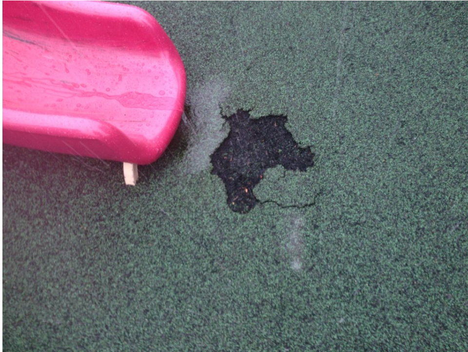
Damage in Poured In in High Traffic Area
