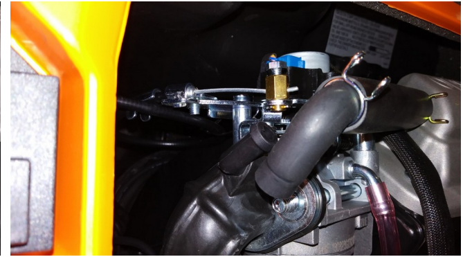
Fig. 5: Breather hose removed from air duct.
