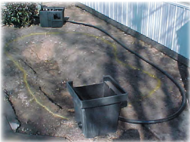
Here we are redoing a small pond in front of a business. The previous pond did not have a skimmer or AquaFalls filter. The owners wanted the pond larger and a stream added. Note the shape has been painted and skimmer, filter and pipe are in position.
