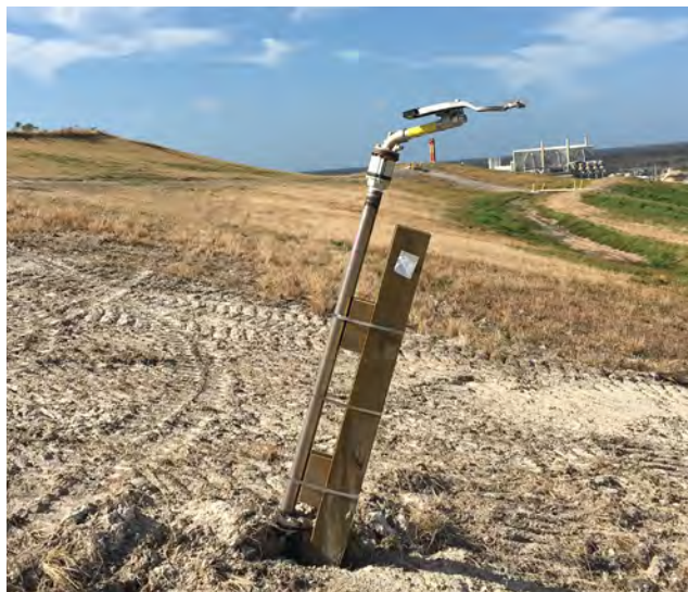
Figure 16. Risers should not be installed perpendicular to field slope. The sprinkler in this photo will have uneven watering and may stall without the use of a counterbalance kit.
