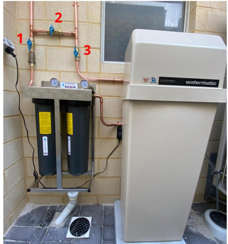
Figure 1. Set Up for filtered water going into your house. Valves 1 and 3 remain open. Valve 2 remain close.
