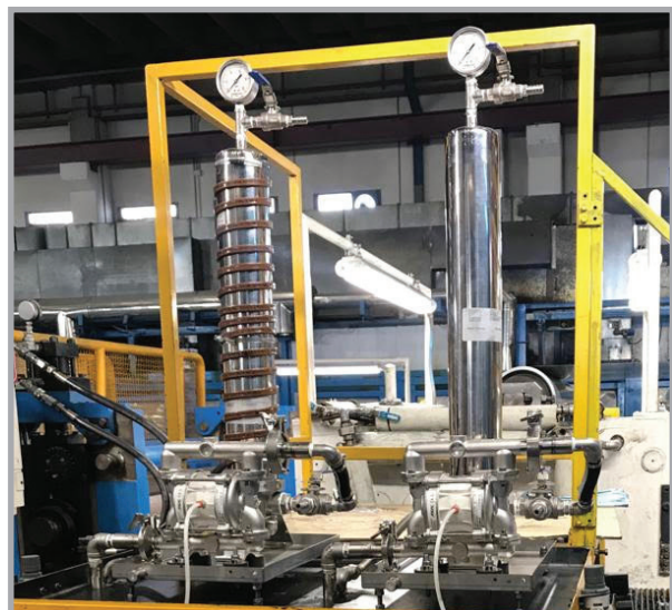
ASTRAevo FOOD (DDE SPN 30) installed in a pharmaceutical plant in Europe.
