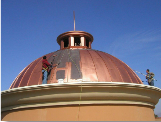
Left: Cabazon Outlet Mall - Cabazon, CA. Coated with Copper B Metal Coating.
