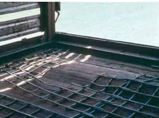
Steel mesh for reinforcing concrete is too light and tends to break up.
