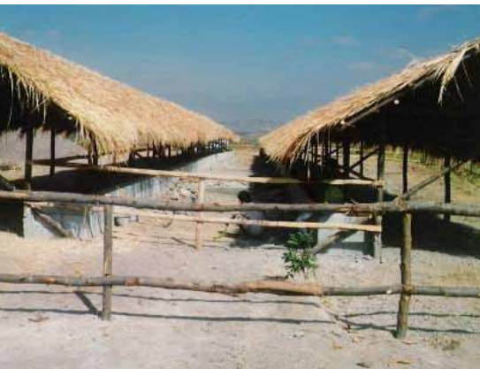
Roofing should provide shade for stock and protect troughs against rain.
