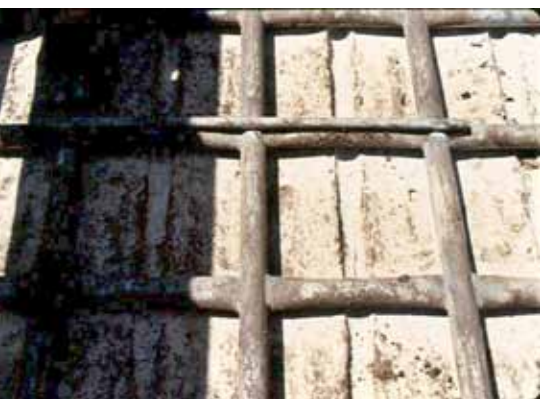
Welded pipe cleats provide good footing and reduce slipping and injuries.
