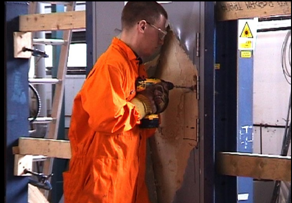
With the door skin removed, a drill is used to attack the hardware.
