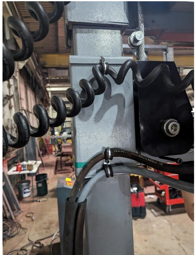
Picture 8.1 Cable and hose ran through loop clamps.
