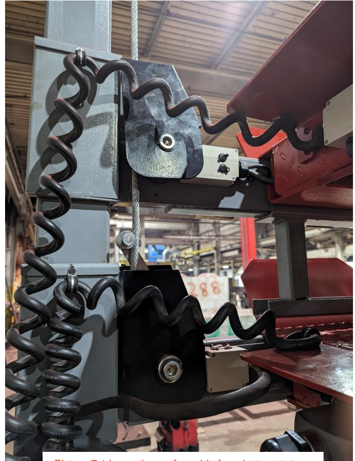
Picture 7.1 Loop clamps for cable from bottom to top runway
