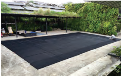
1) Laying out of the panels and marking the design pattern according to the approved design.
