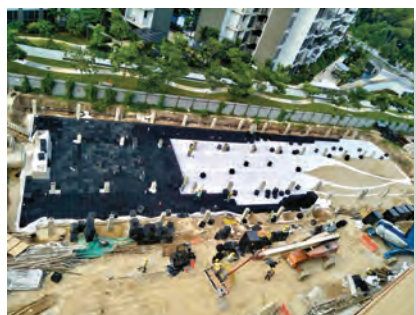
4) Subsequent laying of the PlanterCell® SW Tank. The tanks are secured beside each other using cable ties.
