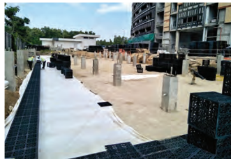
3) Laying of the Insu® Felt geotextile at the tank base and PlanterCell® SW Tank perimeter.
