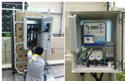
5) Installation and setting of Auto-Irrigation accessories. (e.g. pressure regulators, solenoid valves, controller, etc.)
