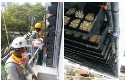
7) Checking and water testing of the irrigation pipes and emitters prior to plant installation.
