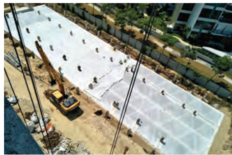
9) A sand layer will be also laid on top of the tank to filter rain water percolating from the carpark floor.
