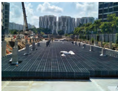
5) PlanterCell® SW Tank laying completed. The Insu® Felt geotextile upturn are bonded on the sides of the tank with adhesive.
