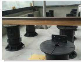
2) Measuring and testing the floor levels & height before securing the wood batten.
