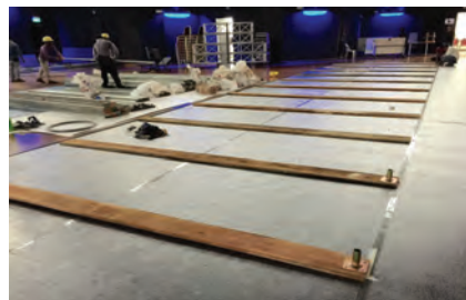
5) At the site, the floors are marked prior to installation of scaffold frame.
