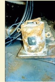
GAUGE PAINTED OVER
