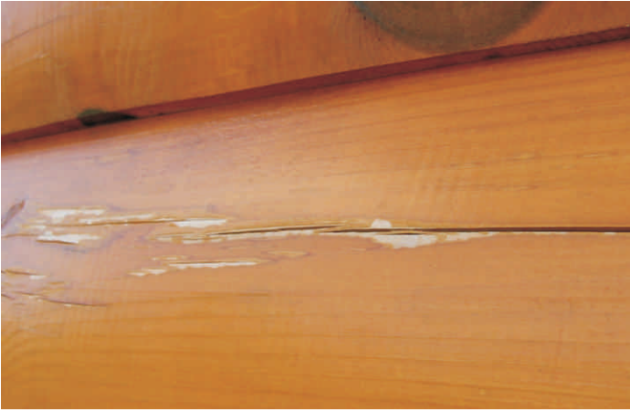
Peeling issue around fissures that formed on surface after application of the finish.
