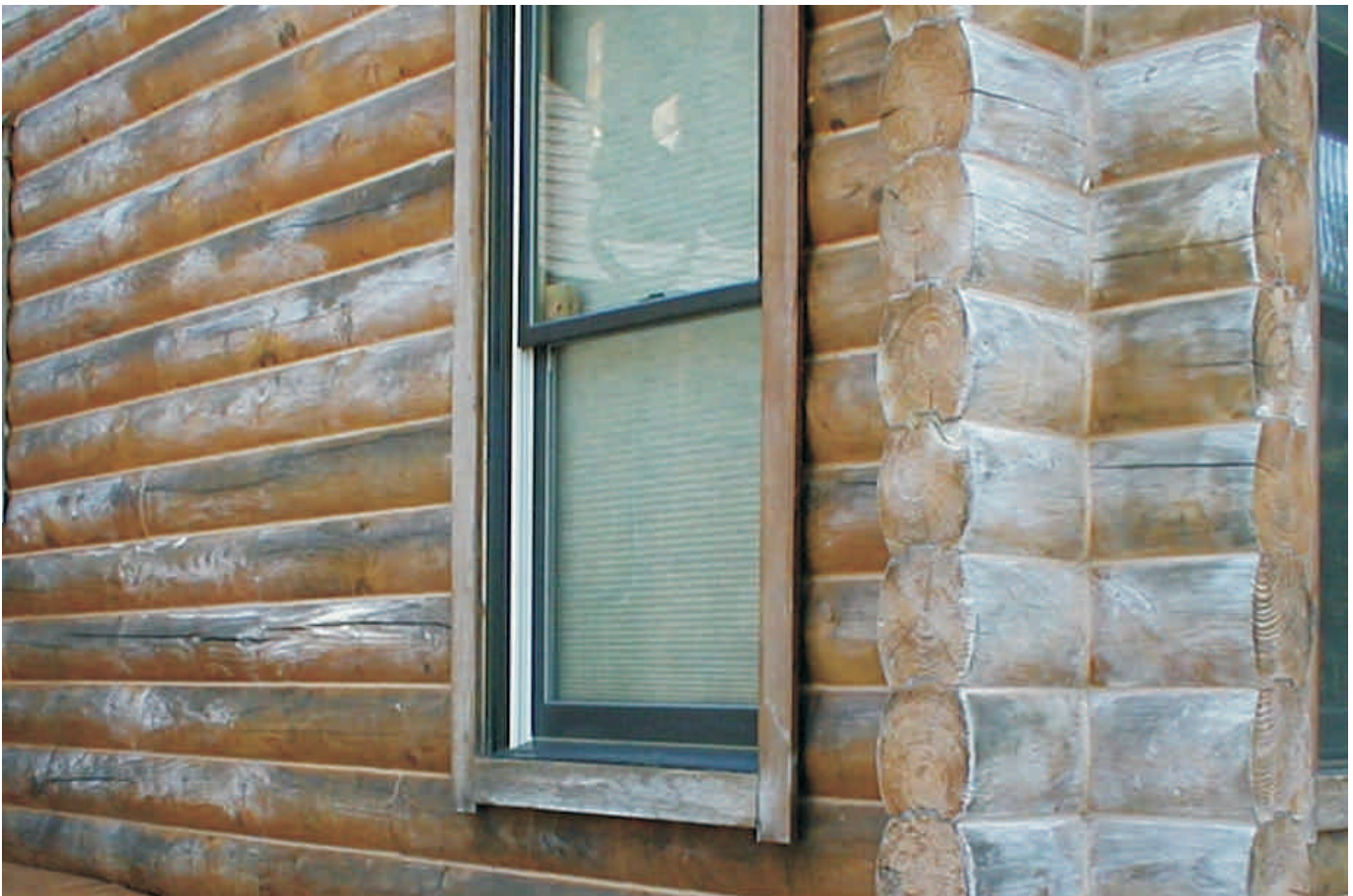
Inadequately mixed Advance Satin applied to home.
