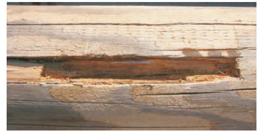
Cleaned out decayed pocket with some loose wood fibers.
