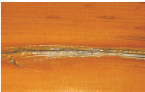
Fissure with peeling.
