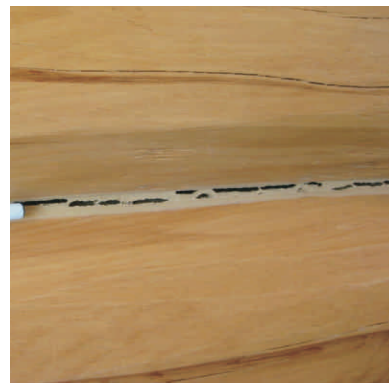
Sealant applied to a narrow seam without backing material.
