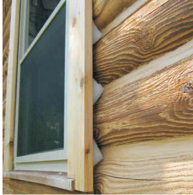
Insert foam blocks into void between logs and frame. Leave 3/8" gap between surface of foam and edge of frame.
