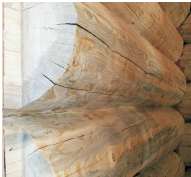
Blue stained logs in a wall
