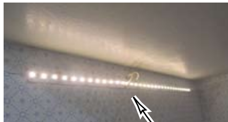
Success! Do not connect the wires to the striplight where it goes over the tapewire
