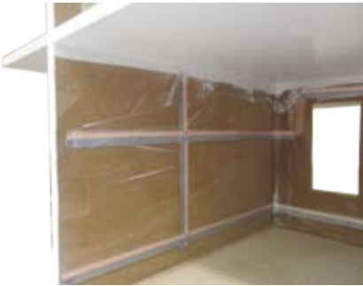
A thoroughly wired house (the Sconce Run will not be used). Note the blue lead is toward the back on the vertical tapewire.
